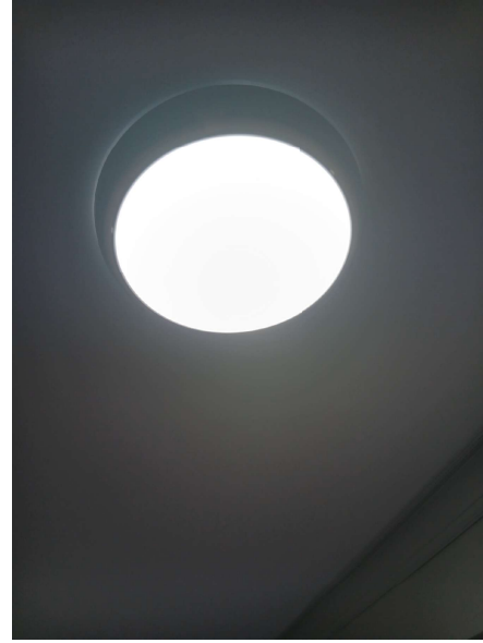
Lighting (Standard and Emergency Lights)
